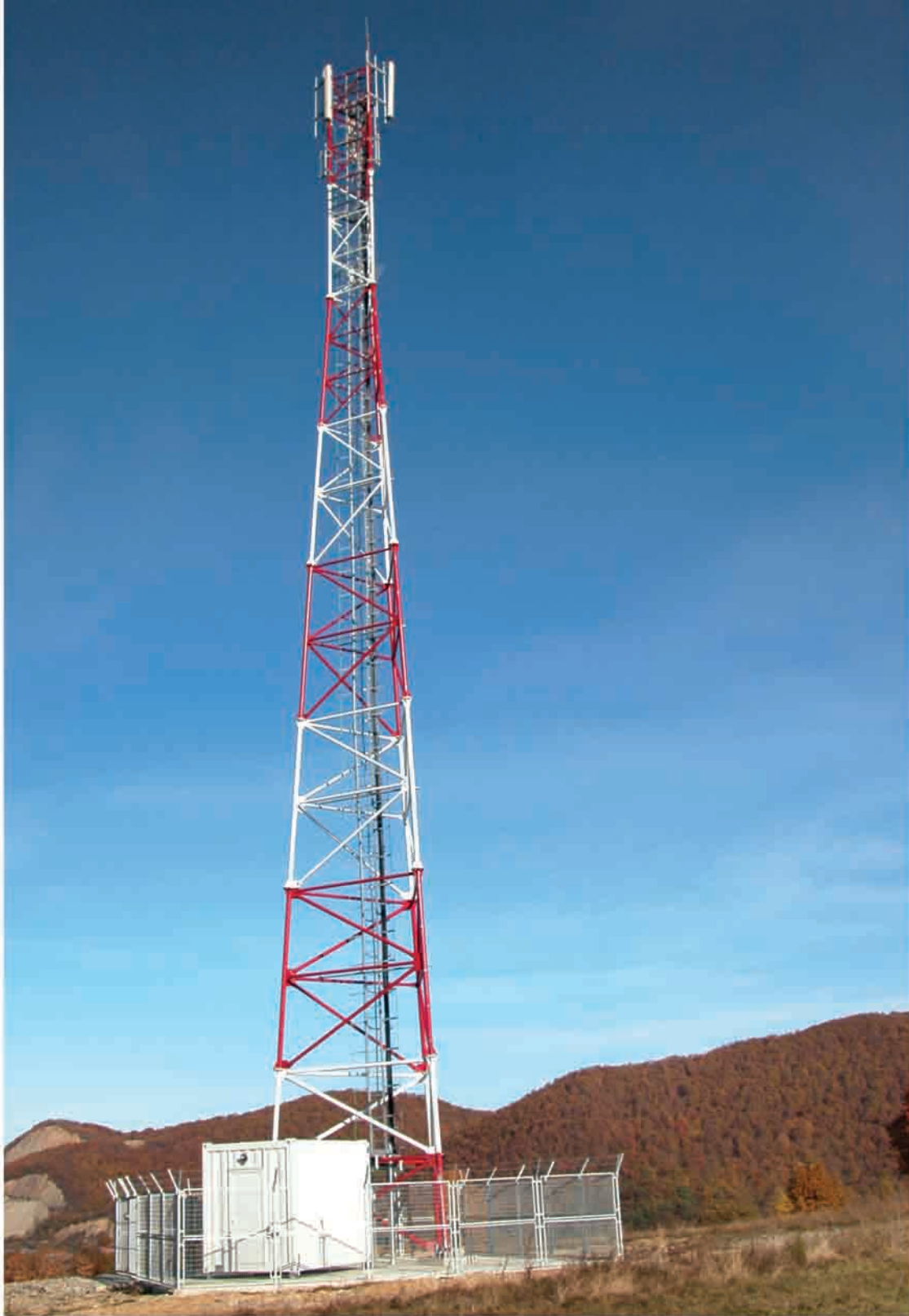
One of the regional telecommunications sites equipped with NFC48S
